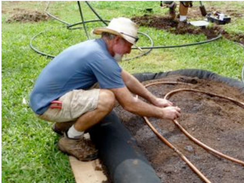
Professional landscapers (Mark Waterbury pictured here) helped us install the irrigation system.
