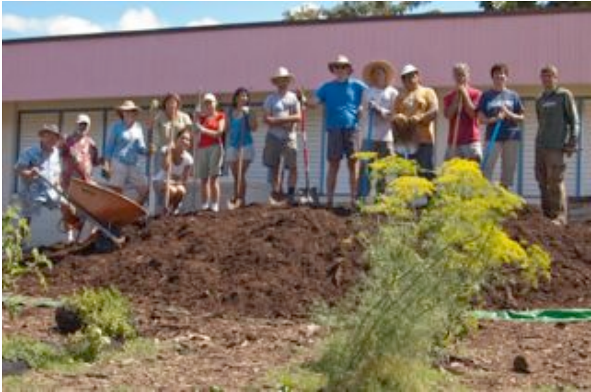
The garden was built in two phases. Over 60 volunteers spread over 86 cubic yards of mulch and cardboard, installed a tool shed, and built a variety of raised beds.
